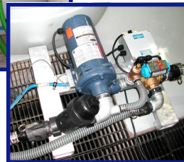
500 Gallon Storage Tank (feeds our computer controlled pump system)
